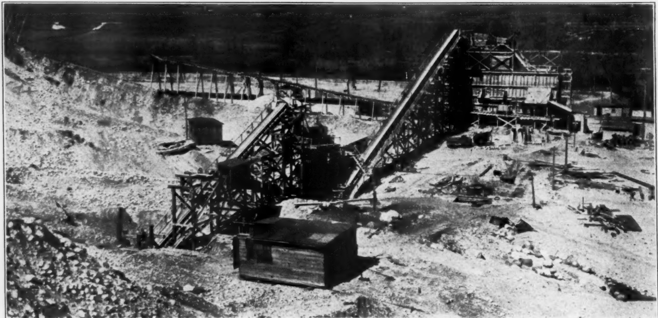
View of the Rebuilt Plant Showing Conveyors to Crusher First and then to Screens and Bins
